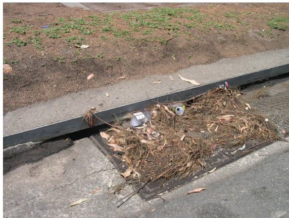
Photo 8 –stormwater grate blocked following a minor storm
