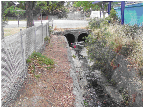
Photo 7 – Example of recent debris blockage at culvert
