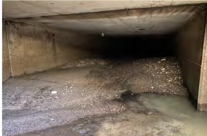
Photo 8: Sediment build up in a culvert
